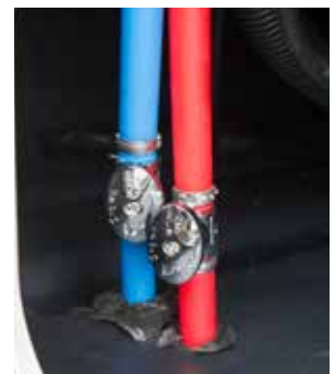
Typical low-point drain valves
