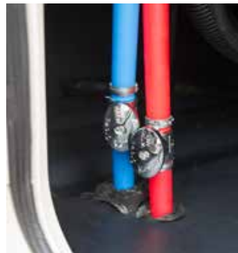
Typical low-point drain valves
