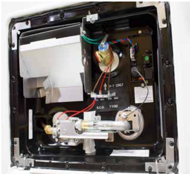
Water heater controls accessed from an exterior cover
