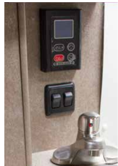
Tank-less water heater User Control Panel (UCP) mounted on a bathroom wall
