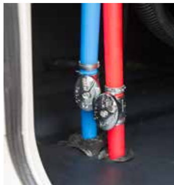
Typical low-point drain valves
