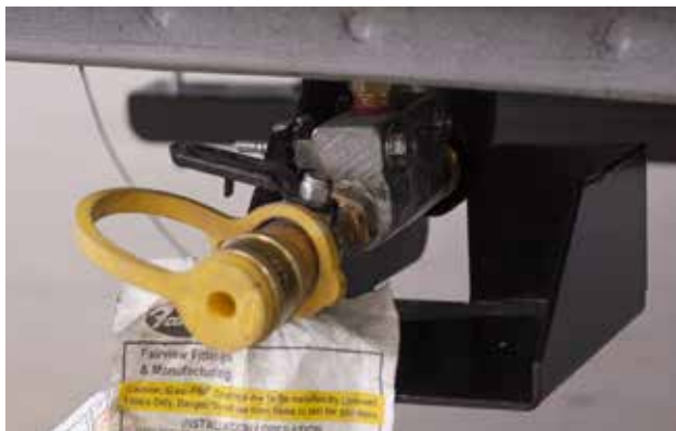
External propane hook-up
