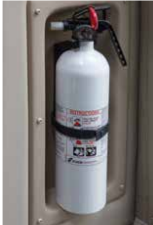
Typical Class B-C fire extinguisher
