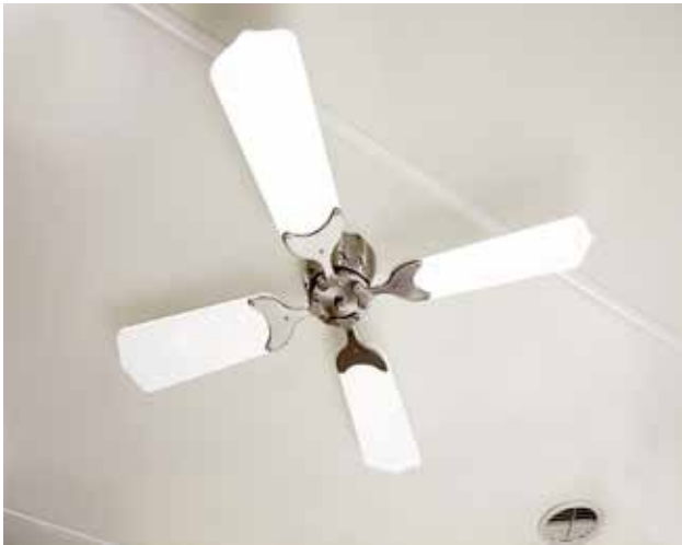
Typically, paddle-type fan installed in the ceiling of a bedroom
