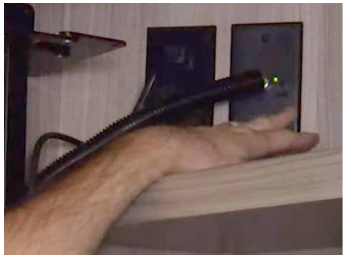
Typical antenna/cable switch panel (or booster plate)
