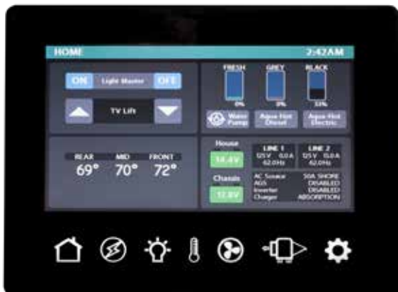
Typical multiplex main control panel. Electrical system monitoring is usually located on the main menu (House) screen.
