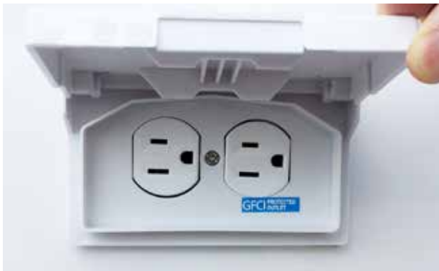
Typical outside 120 volt AC receptacle
