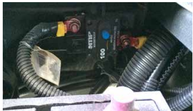
Typical Inverter Circuit Breaker
