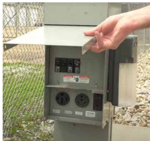
Typical Campground electrical service stand. This illustration shows 50 amp, 30 amp, and 15-20 amp outlets, along with corresponding circuit breakers.
